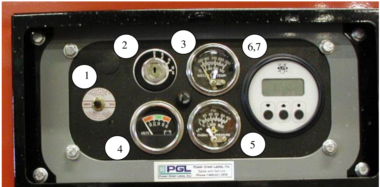
(Typical Control Panel)
